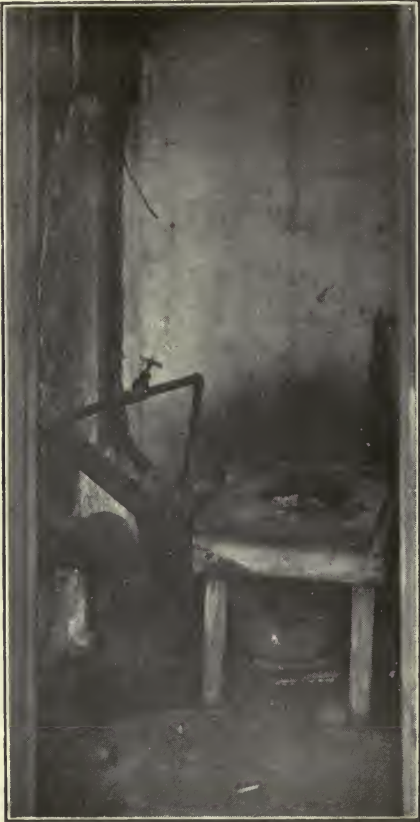
This unique cellar closet is "flushed" by turning on the faucet
